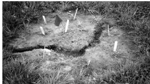
Gopher damage in revegetation area
